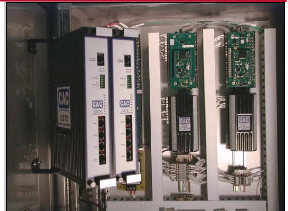
The CS7X wellsite manager monitors and logs subsurface data from the sPOD gauges.
