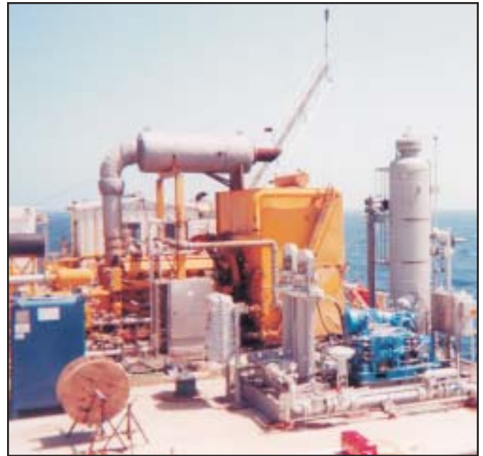
Weatherford 10x42 RamPump system at EI 257D in operation since April 2001.
