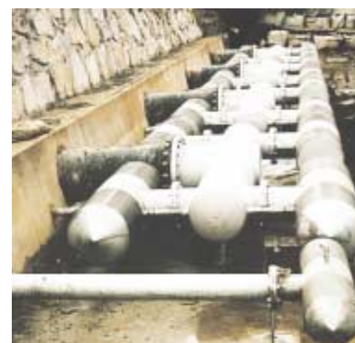
Intakes connected in parallel
