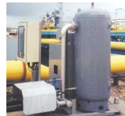
Control panel receiver tank
