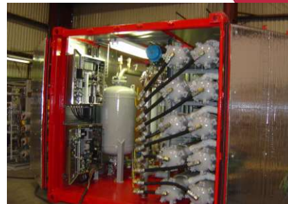
Internal View of a Containerized Nitrogen Generation System
