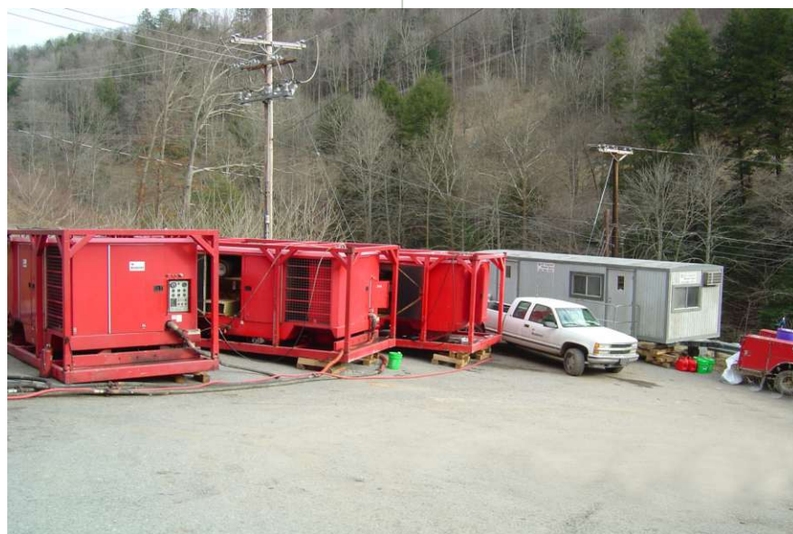
Compression and Nitrogen Units on Site at Thermal Event in Virginia
