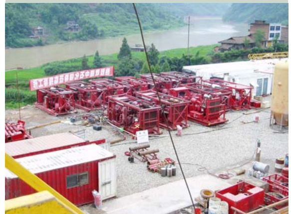
Weatherford 6,000 scft/min air package rigged up on location in Puguang, six compressors, three boosters, and a mist pump.
