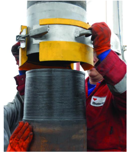
An 11 3/4- × 13 3/8-in. MetalSkin monobore openhole liner extended the 13 3/8-in. casing and enabled an 11 3/4-in. long string to be set and cemented below the expanded liner.
