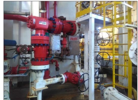
HPFM skid in Standpipe #1 (SP#1).
