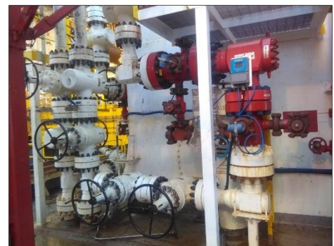
HPFM skid in the booster line.
