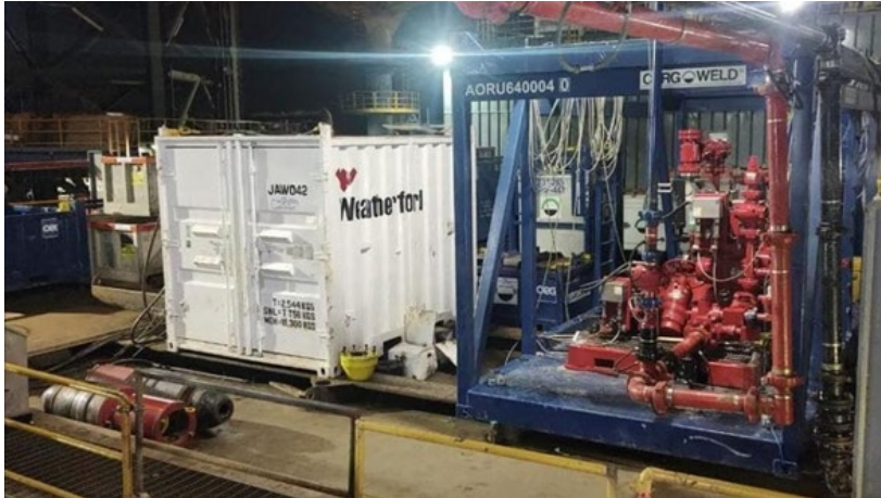
The MPD equipment, including the Modus solution, rigged up on the jackup rig.
