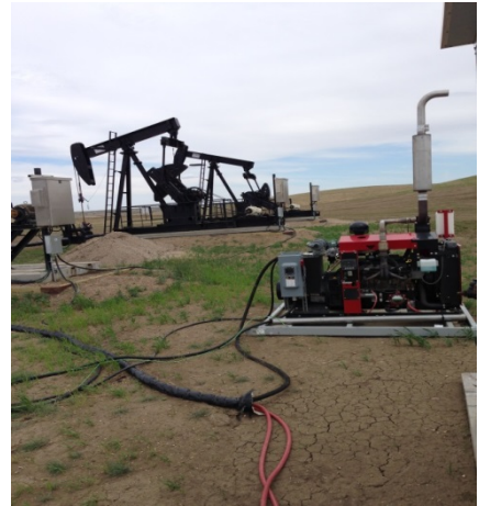
The Weatherford GM 5.7 44-kW power generator equipped with IEPR technology enabled the client to significantly reduce propane fuel consumption.
