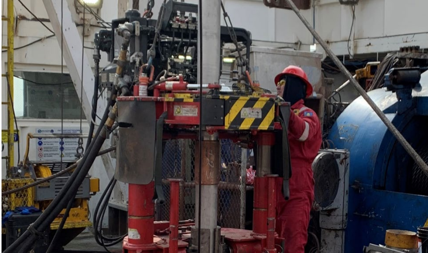
The Vero system requires only one person on the drill floor to reduce personnel exposure in the red zone.
