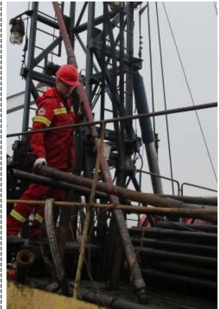
The crew ran the MetalSkin cased-hole liner expansion system into the well with minimal loss of inside diameter.
