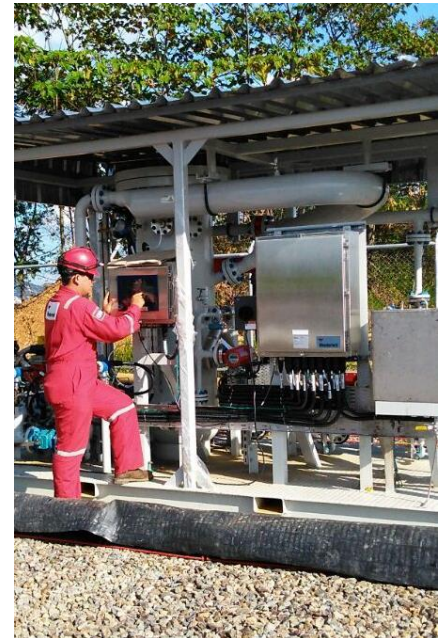
The compact Red Eye multiphase flowmeter system reduced the average single-well test time by 72 hours.
